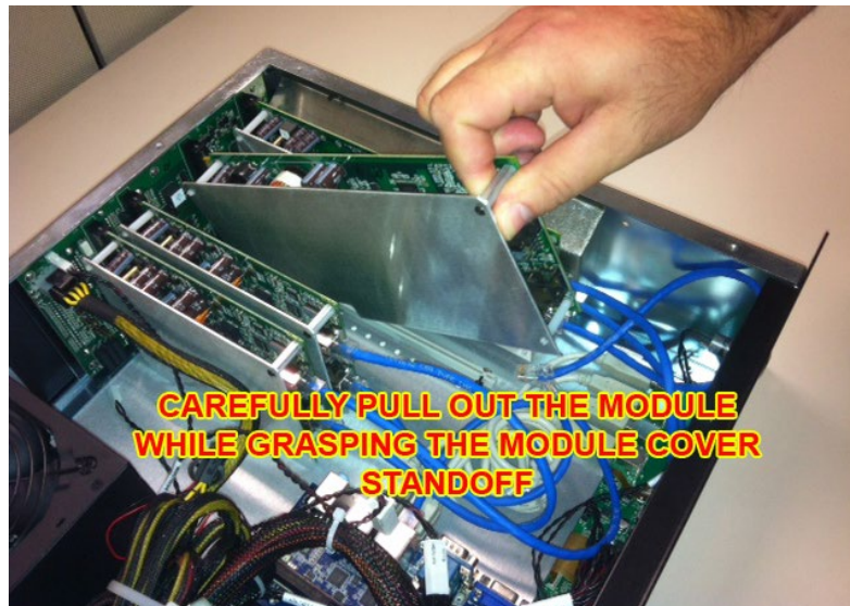
Figure 13-5 Removing the Control Module from the EBC Chassis
